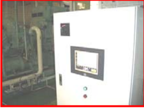
Low Air compressor auto operation
