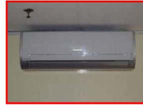
Convert split air-cond to inverter type
