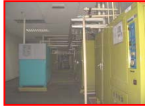
Install individual chiller for Plastic Injection machine
