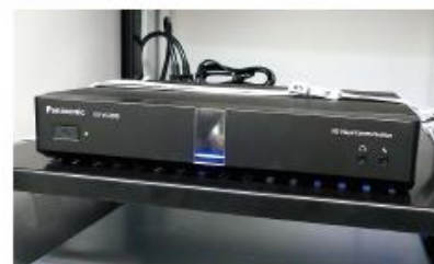
HDVC main unit (KX-VC2000J) installed in the head office server room
