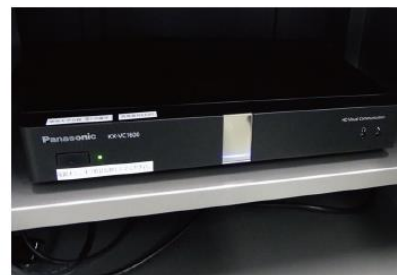
HDVC main unit (KX-VC1600J) installed in a designated box
