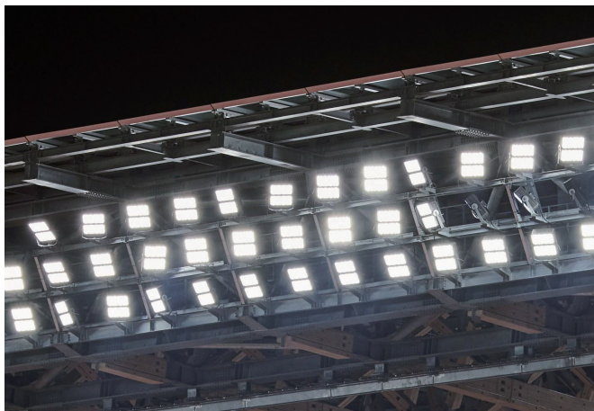
LED floodlights use light sources that accommodate color reproducibility in shooting for TV.
