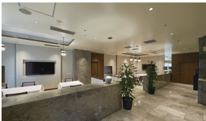
LED downlights in operation at the suite restaurant in the corporate area "THE SUITE TOKYO".
