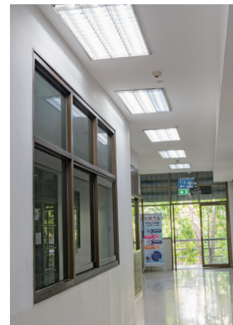
Lights in the hallways are also automatically turned on when the sensors detect human presence, and the lights are automatically turned off when no one is there.
